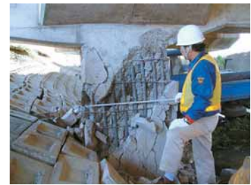
Damage to an elevated Shinkansen bridge from the Chuetsu Earthquake (2004)
