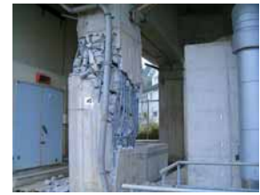
Photo 2. Earthquake-induced fracture of a Shinkansen pier
