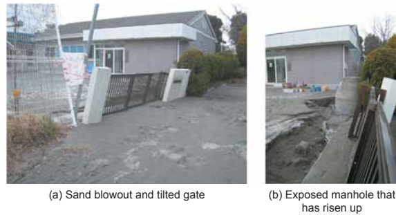
Photo 1. Damage from liquefaction (Urayasu city)
