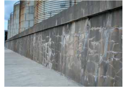
Retaining wall exhibiting the effects of the alkali-silica reaction
