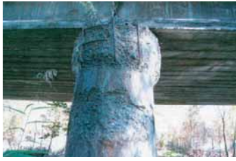
Pier revealing frost damage
