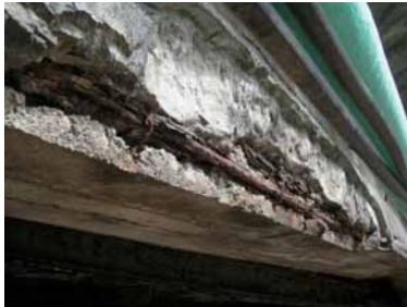
View from below of a bridge damaged by chloride attack
