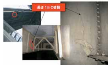
Photo 2. Yamazoe Bridge (fatigue crack)
