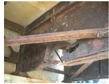
Photo 3. Benoki Bridge (corrosion)
